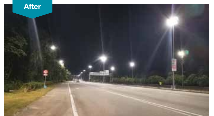
The addition of LED street lighting to our highway mainlines has improved night time visibility at all our highways.
