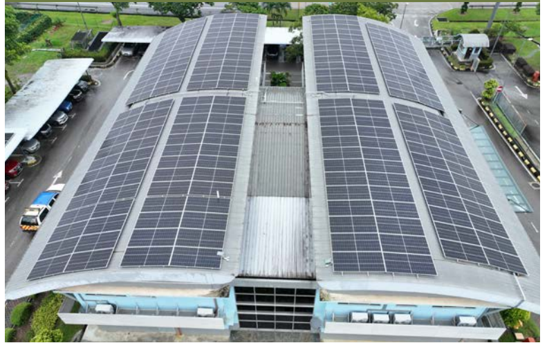
➡ Rooftop solar PV installed at Elmina Toll Plaza, GCE.
