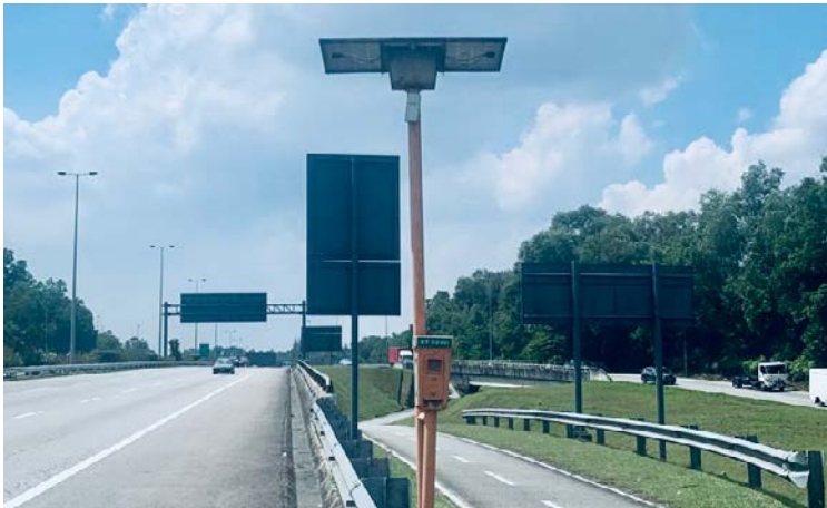
→ Solarised Emergency Telephone at GCE.
