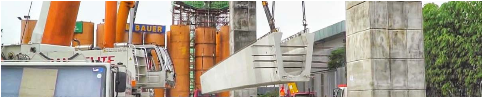
➡ SUKE and DASH structures are constructed using the Industrialised Building System (IBS) technique.
