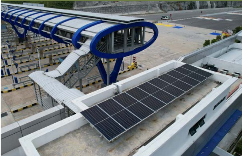
➡ Rooftop solar PV installed at Bukit Teratai Toll Plaza, SUKE.
