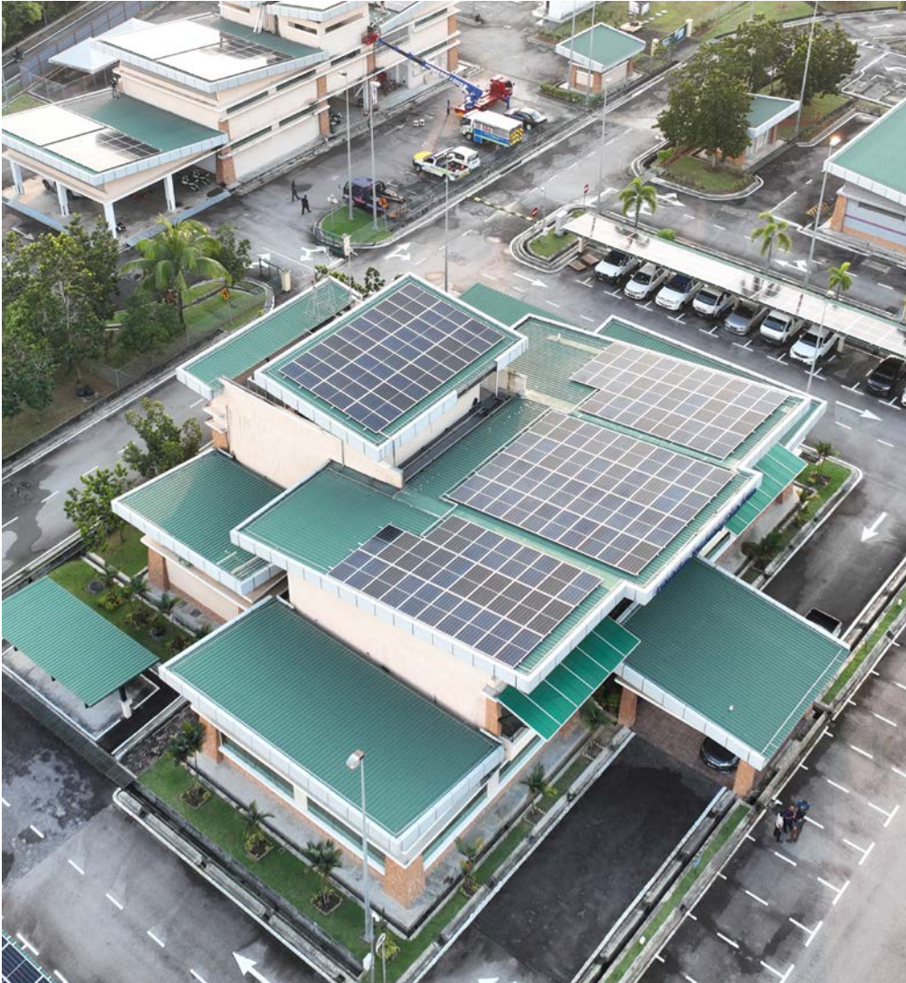
→ Rooftop solar photovoltaic panels installed at LKSA's Administration Office Building.
