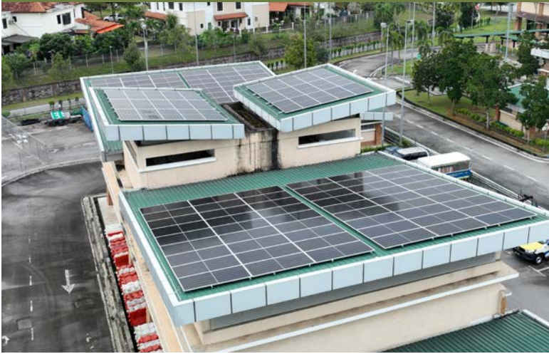
➡ Rooftop solar PV installed at Alam Impian Toll Plaza, LKSA.
