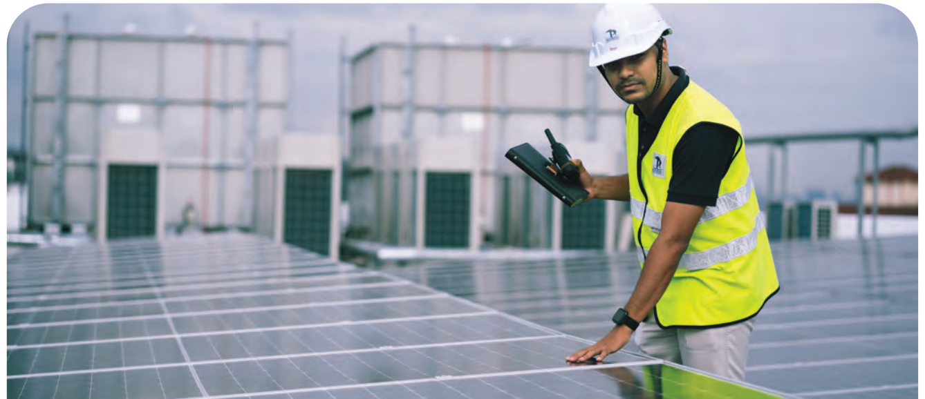
Harnessing solar energy at SUKE's Alam Damai Toll Plaza – sustainable, efficient and cost-effective.
