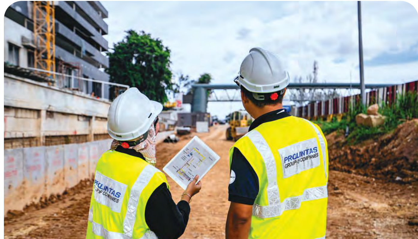
The Pipe Jacking Technique minimises the negative impact on the environment and disruptions to traffic due to its non-evasive technology.
