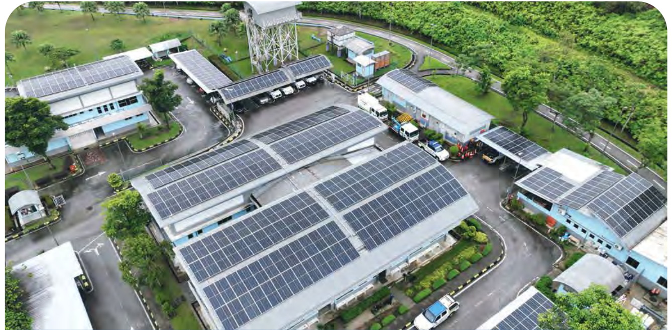
Powering up the GCE's office building with solar energy.
